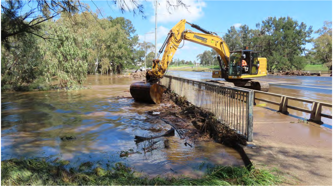
Figure 6: Litter and debris being pushed downstream from Serisier Bridge in October 2022 (photo: Ken Smith)
