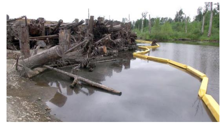
Using 'nature-based infrastructure', such as log-jams, the project engineers are able to reduce flooding and benefit salmon. Photo: NOAA.
