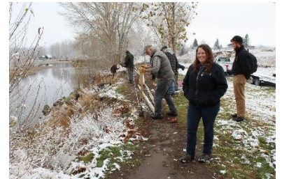
Digging post holes for protective fencing in the snow – the dedication of volunteers. Photo: Michelle McConnaha.
