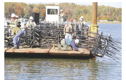
A barge-load of fish habitat ready to be installed. Photo: John Shepelwich.
