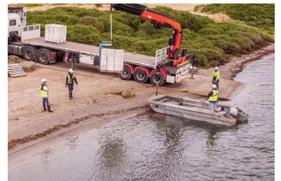
One more pallet of limestone blocks being loaded ready to be installed in the river. Photo: Travis Howson.
