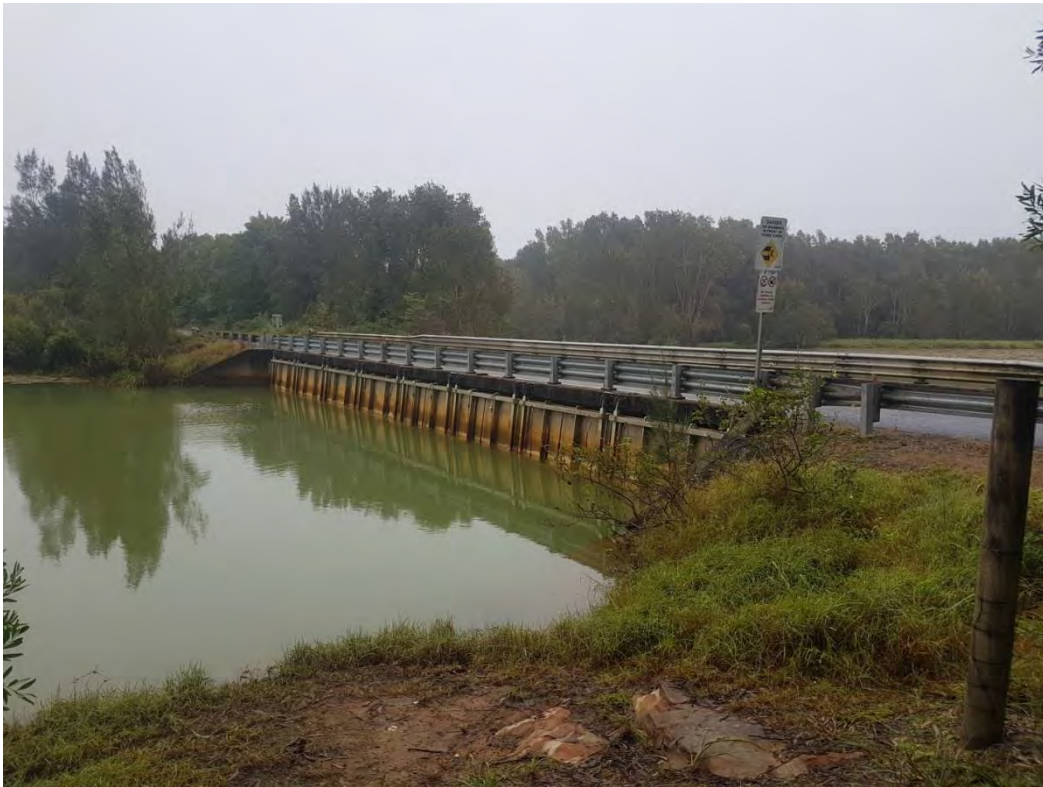
Figure B-5: Bagotville Barrage – downstream control structure of Tuckean Swamp (looking upstream)
