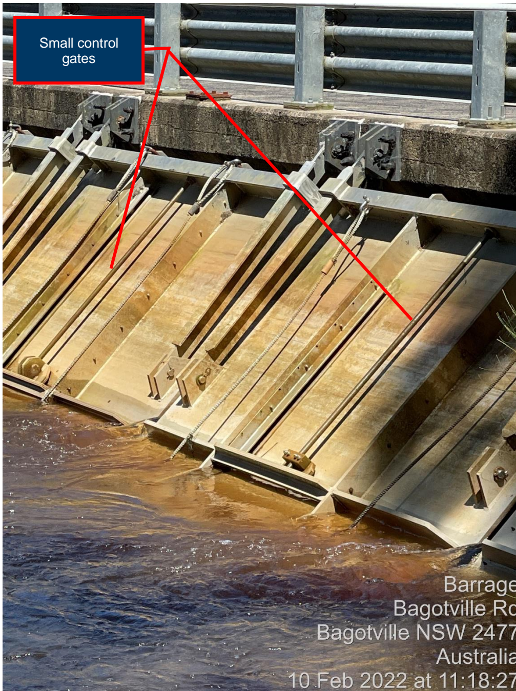
Figure 2.4 Flood gates at the barrage with smaller control gates
