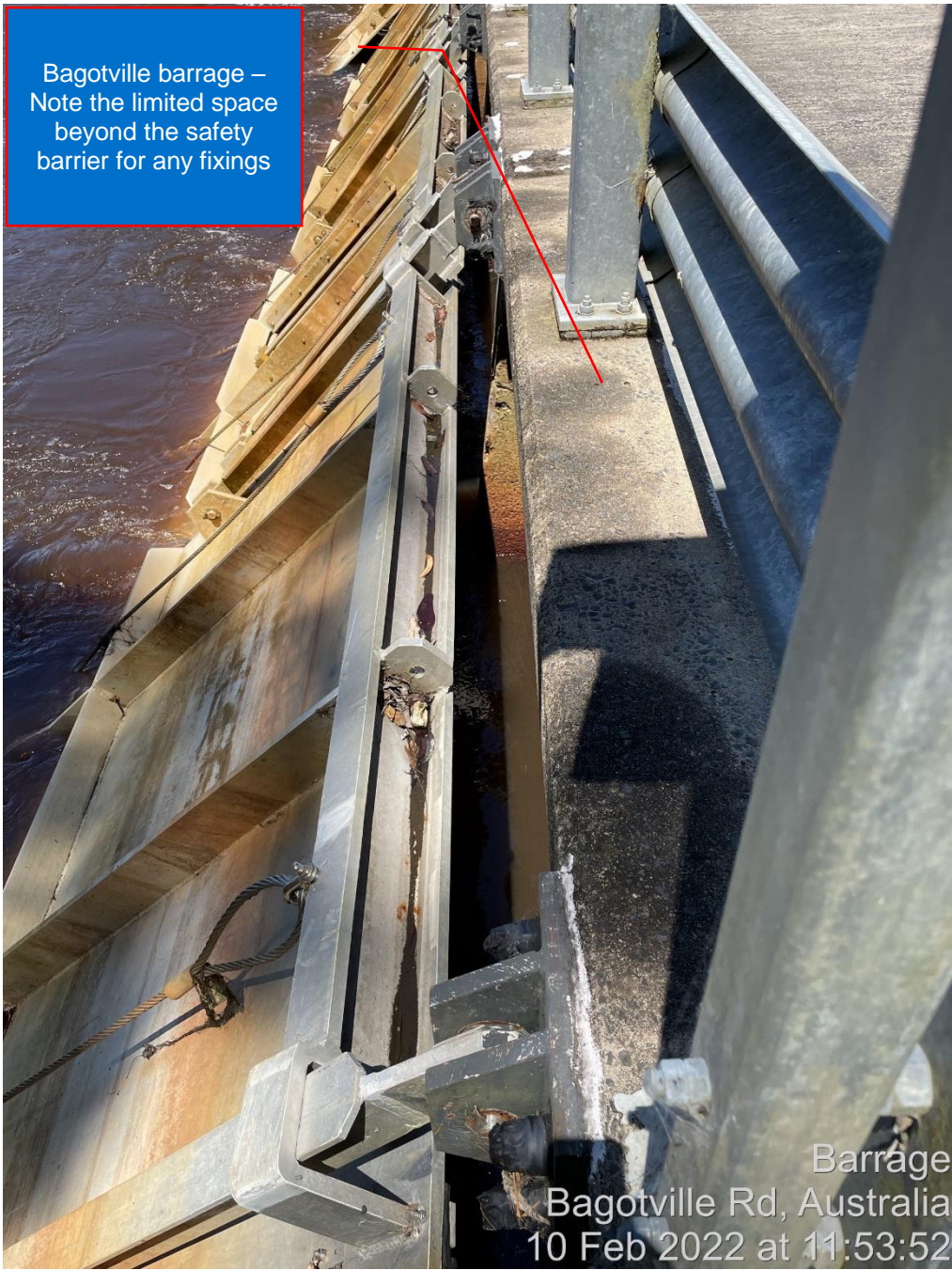
Figure 2.3 Flood gate fixing at the barrage
