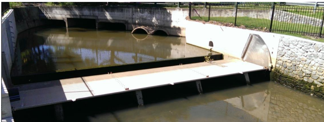
Figure 3.7 AWMA tidal gate (looking from downstream) (AWMA, 2022d)
