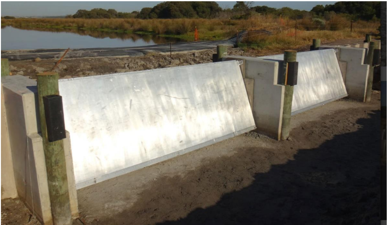
Figure 3.6 AWMA tidal gate (looking from upstream) (AWMA, 2022d)
