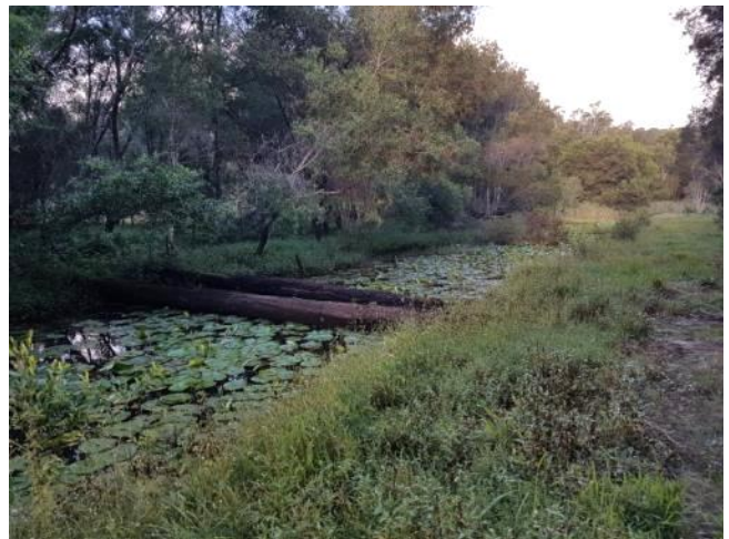
12: Significant blockages of Nature Reserve Drain
